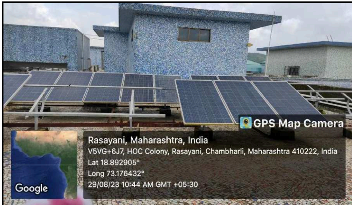
Figure: Solar Panel
