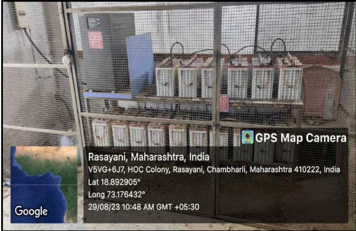
Figure: Solar Battery
