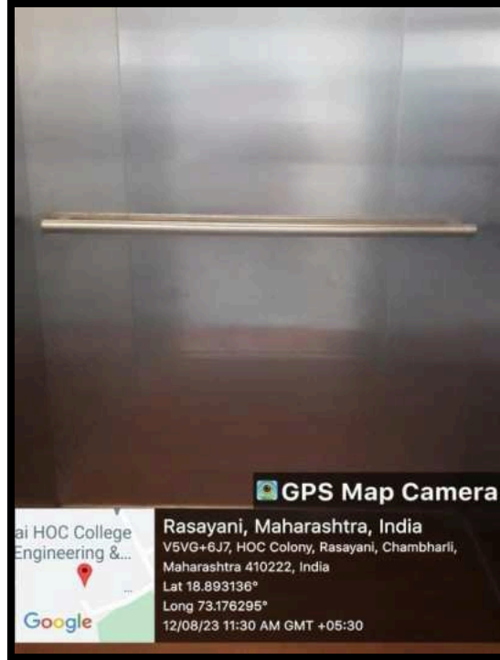
Figure : Handrails in Lift1 for disabled
