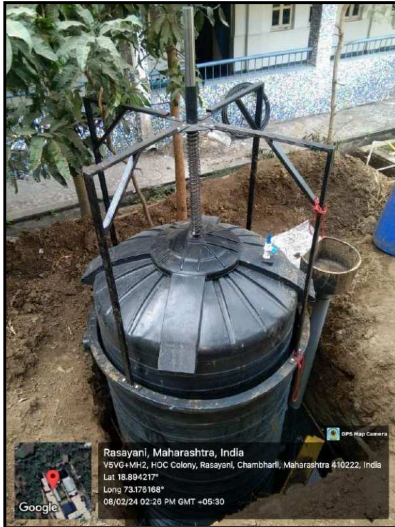
Figure:Bio gas plant
