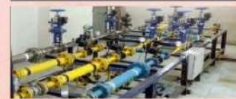
GAS MIXING STATION (GMS)
