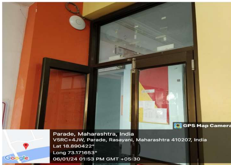
Geotagged photos of Router placed in lab and staff room:
